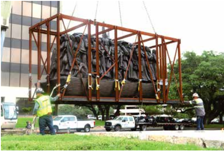
A crane lifts the Angels Unawares sculpture into place on the berm at the Catholic Life headquarters building.
